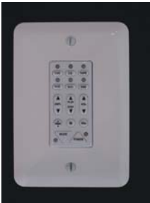
Includes 2 keypads Typically installed In the kitchen & Master Bedroom
